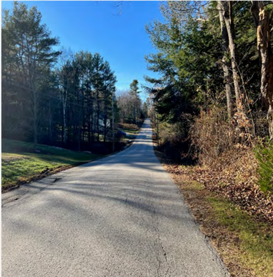
Photo1- Vickery Road Gulley
